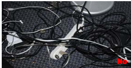
Extension cords shall not be used as permanent wiring
