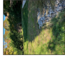
Good Condition Minimal Erosion & Vegetation Intact structure, Adequate size Cleaned of debris
