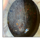
Moderate Condition Some Sediment and Debris Inadequate size, Erosion, Slight structural damage
